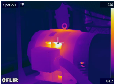
Overheated Breaker Connection
