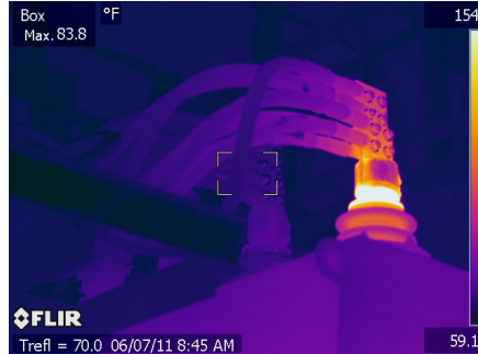
Overheated Transformer Bushing
